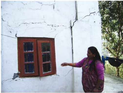
Figure 34: Damaged building above reservoir of 510 MW Teesta V project (Source: Amelie Huber)
