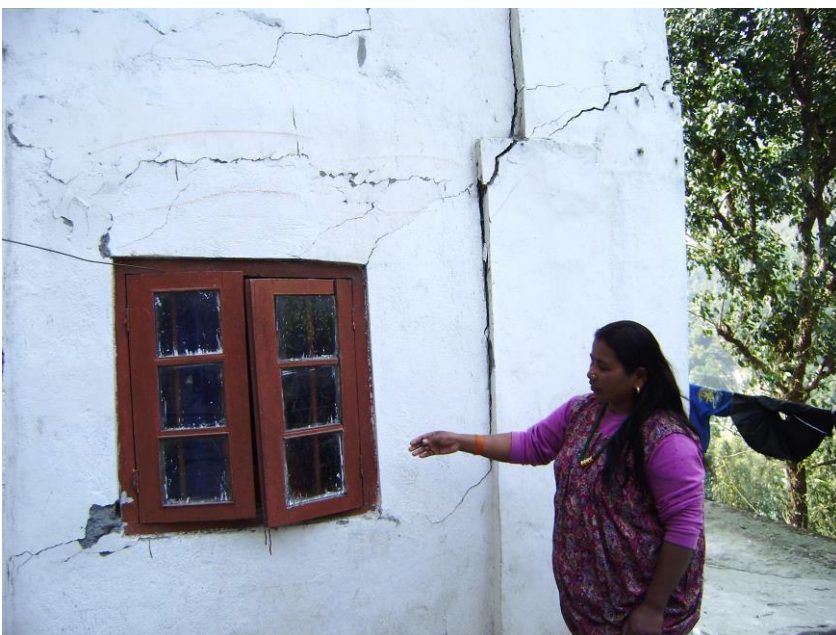
Figure 34: Damaged building above reservoir of 510 MW Teesta V project (Source: Amelie Huber)
